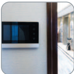
Camera Εισόδου Entrance Camera
