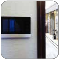
Camera Εισόδου Entrance Camera
